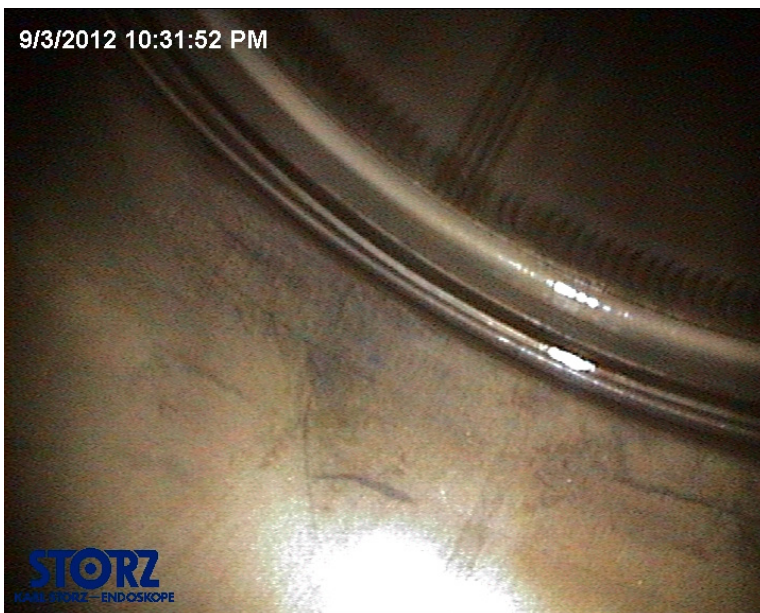
Oil-wetted surface inside the pneumatic manifolds
