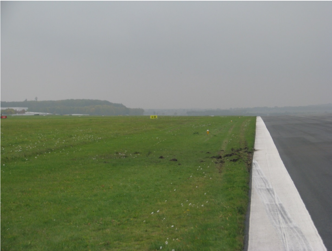
Wheel marks of the right main landing gear veering off the runway
