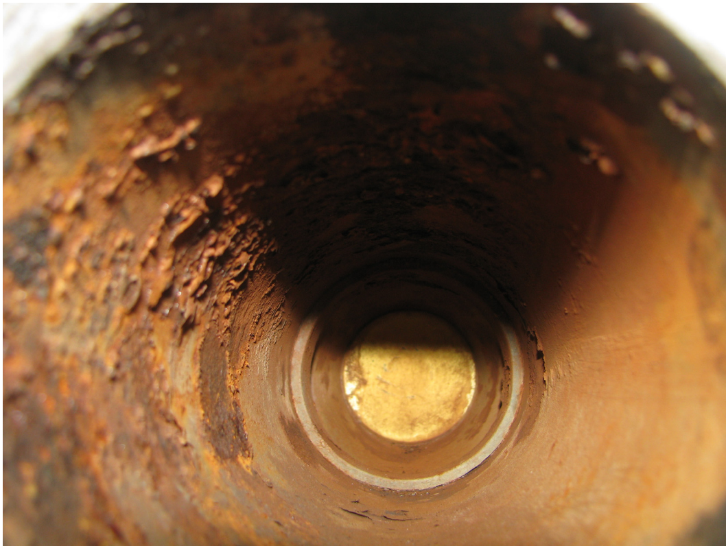
Appendix 7: Corroded inside wall
