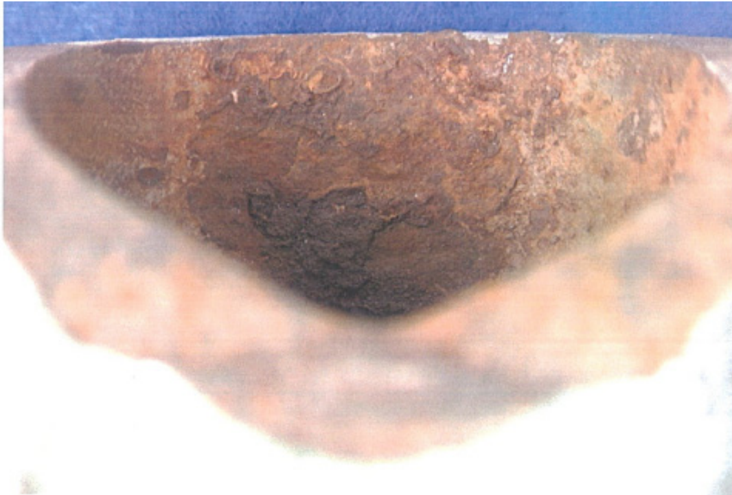
Appendix 8: Corrosion in the 6 o'clock position (top view)
