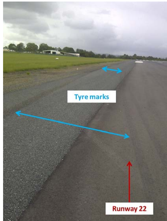
Figure 3: Tyre marks on runway 22
