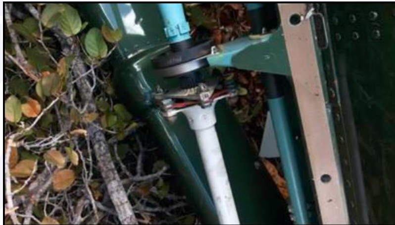
Figure 7 - Coupling of the connecting shaft with the drive shaft of the tail rotor.
