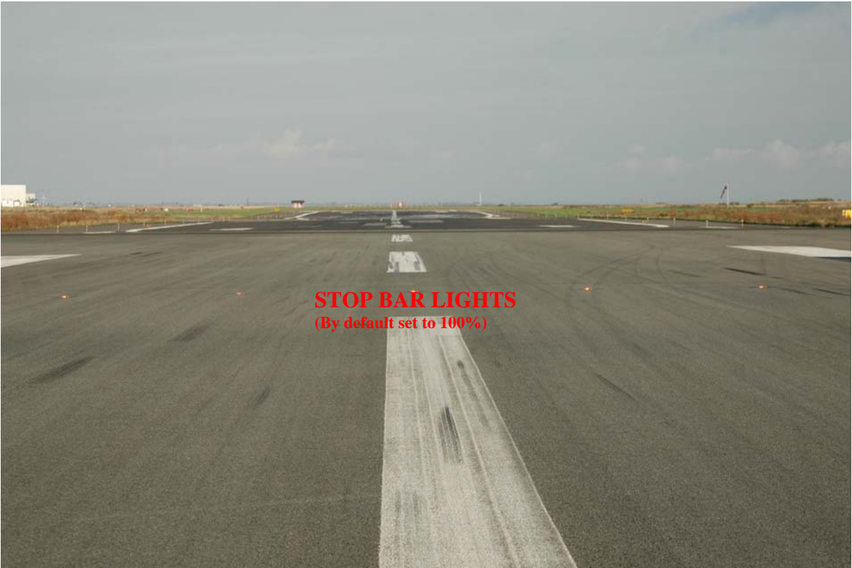
Stop bar and runway guard lights on runway 12
