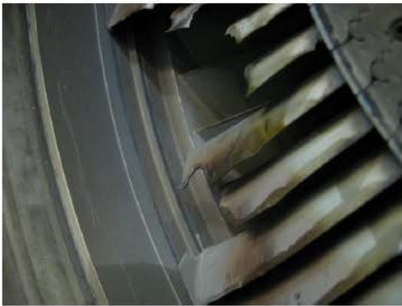
Photo No 13 PT Blade stage 2
