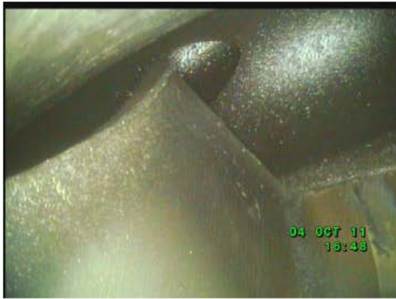
Photo No 7 HP Impeller rubbing
