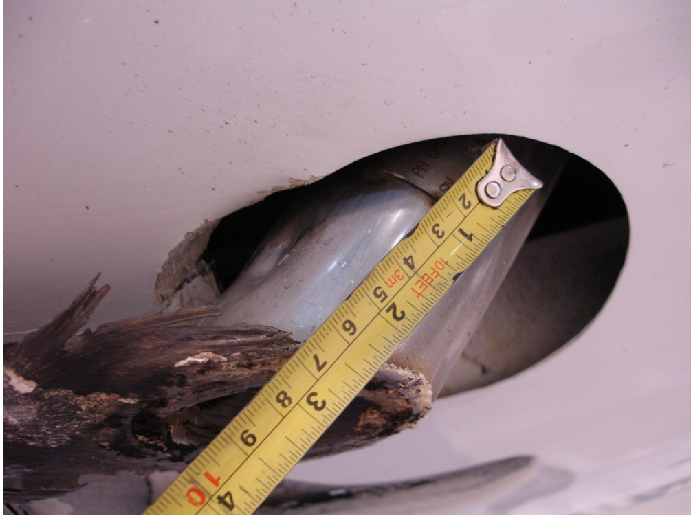
Figure A1-8c : Damaged Right Hand Exhaust Tube with remaining length of 7 cm outside the engine casing
