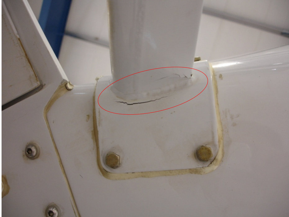
Figure A1-4 : Fatigue Damage on the Root of Left Hand Foot Step
