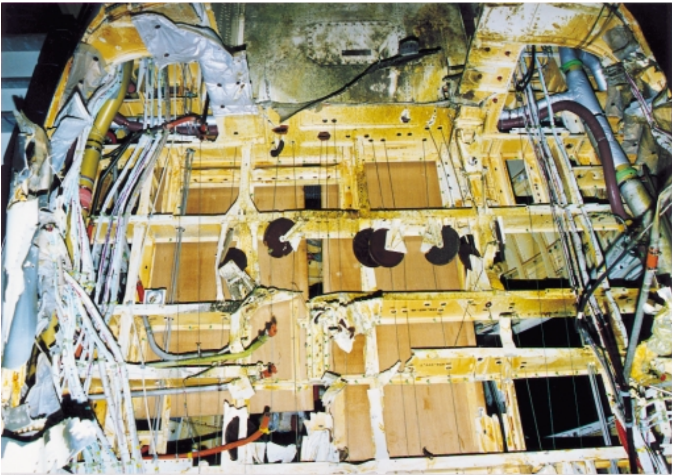
DAMAGE TO CONTROL CABLES
