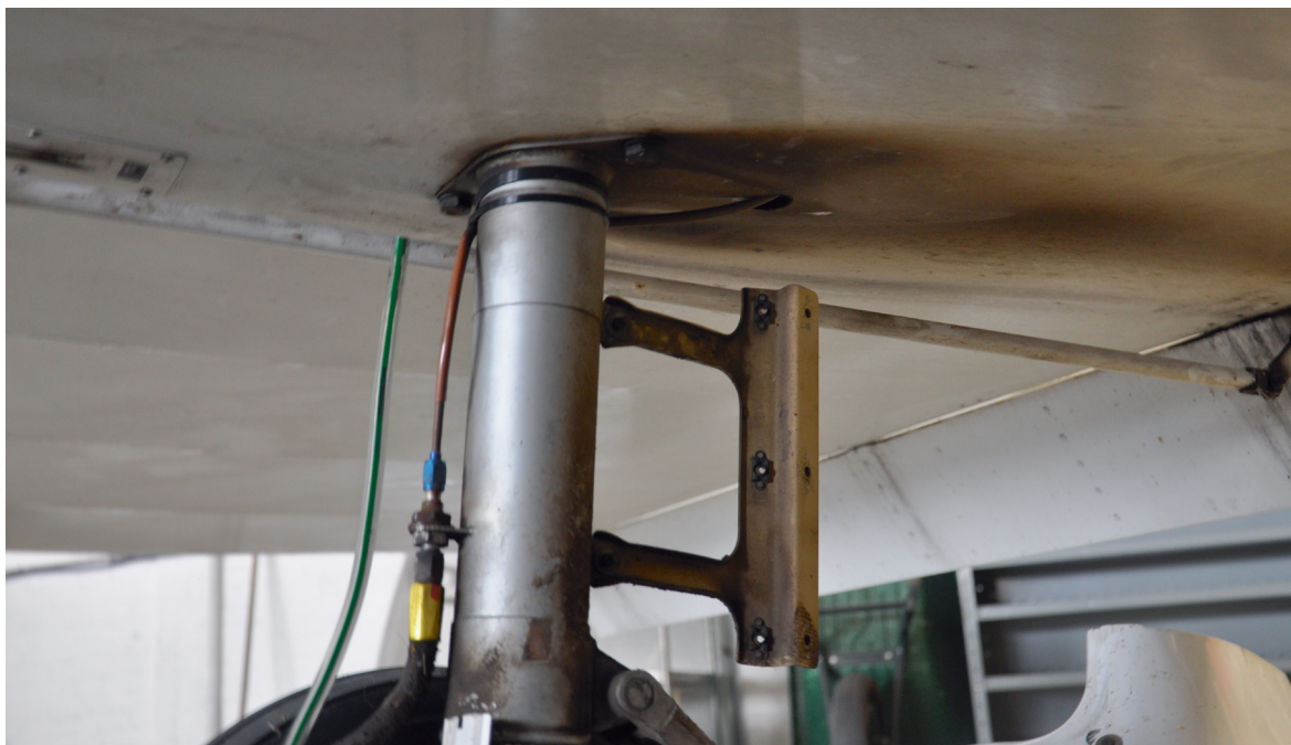
Figure 11: PH-HLR side-view of right-hand gear strut with both fairings removed, showing the dark coloured mark on the wing covering. (Photo: Dutch Safety Board)
