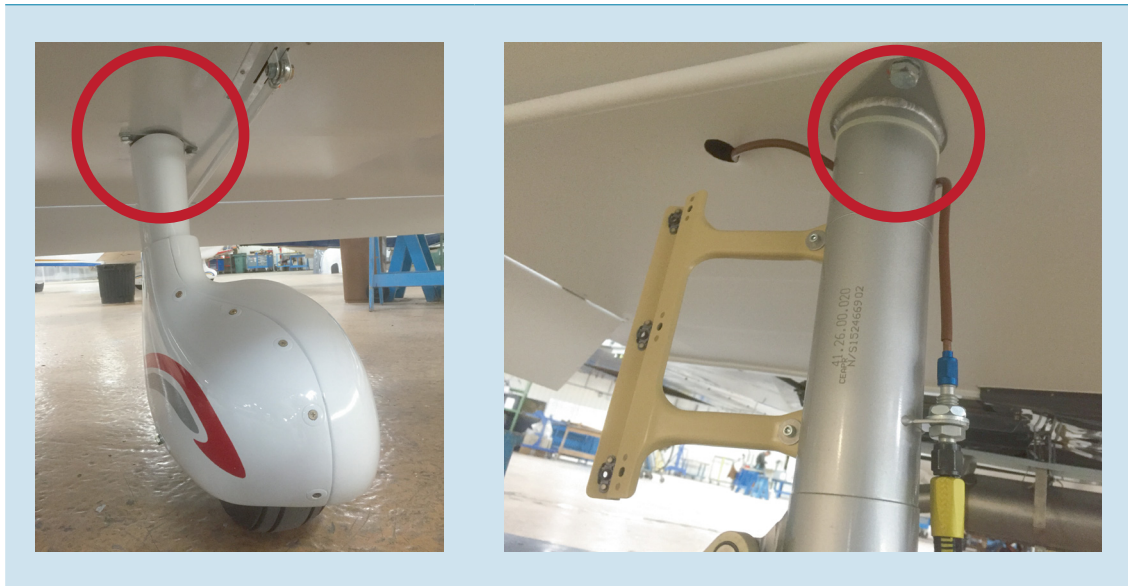
Figure 15: The wing-strut connection plate (marked in red), seen with and without fairing, during construction. (Photos: Dutch Safety Board)
