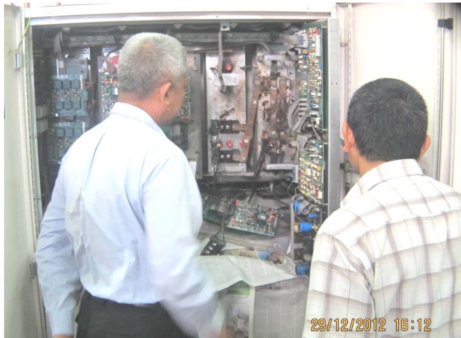
Figure 5: The inverter control terminal after cleaned from debris
