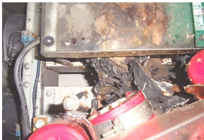
Figure 4: The capacitor materials debris at the inverter control system bus bar
