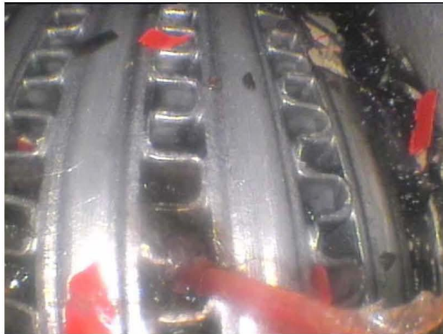
Picture 4: pollution and debris found within the “oil to fuel heater” inlet duct.
